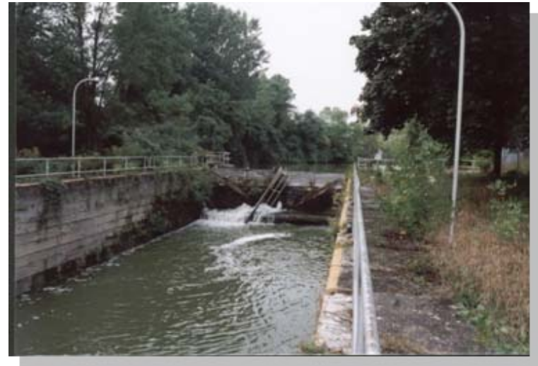
Current Lock in Disrepair
